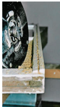
Figure 14. On the lower sash, cut 1/8" by 3/8" kerf on the meeting rail. This is where the barbed-pile will go.
