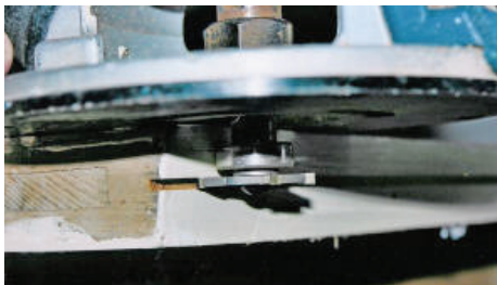
Figure 2. For the upper sash, cut 1/8" by 3/8" kerf on the top. This is where the silicon flap will go.
